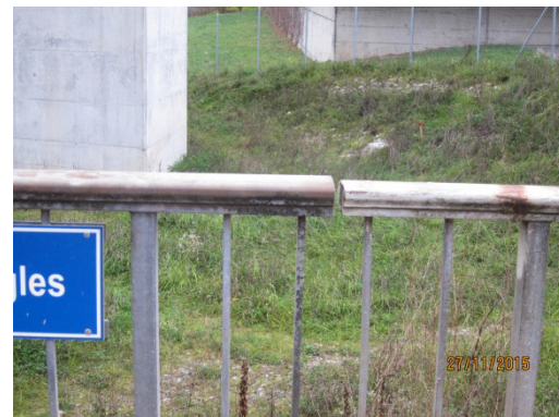
N°12 GARDE-CORPS AVAL CORRODÉ
